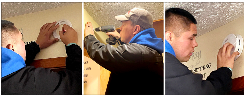
ABOVE, Choctaw Fire Department personnel installed over 50 smoke detectors in the Pearl River community as part of the Sound the Alarm initiative on Friday, Jan. 19.
