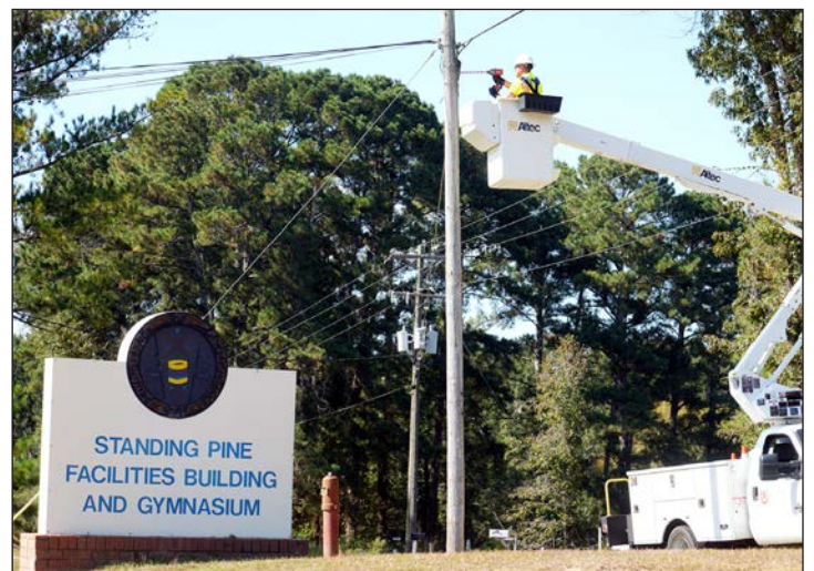
Contractors are currently in several Tribal communities connecting broadband wiring & fiber optics to provide access for 650MB/sec broadband service by MaxxSouth Broadband.
